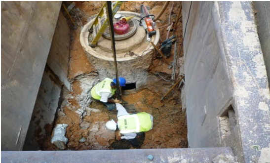
Onsite Engineering Support for Capacity, Management, Operation and Maintenance
